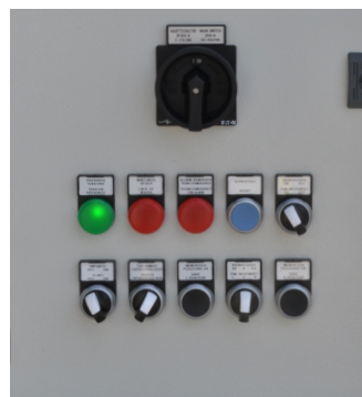
Control panel of industrial dust control system Rino
